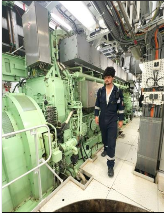
Figure 5: Pre-Departure Checks (Diesel Generator 1)
