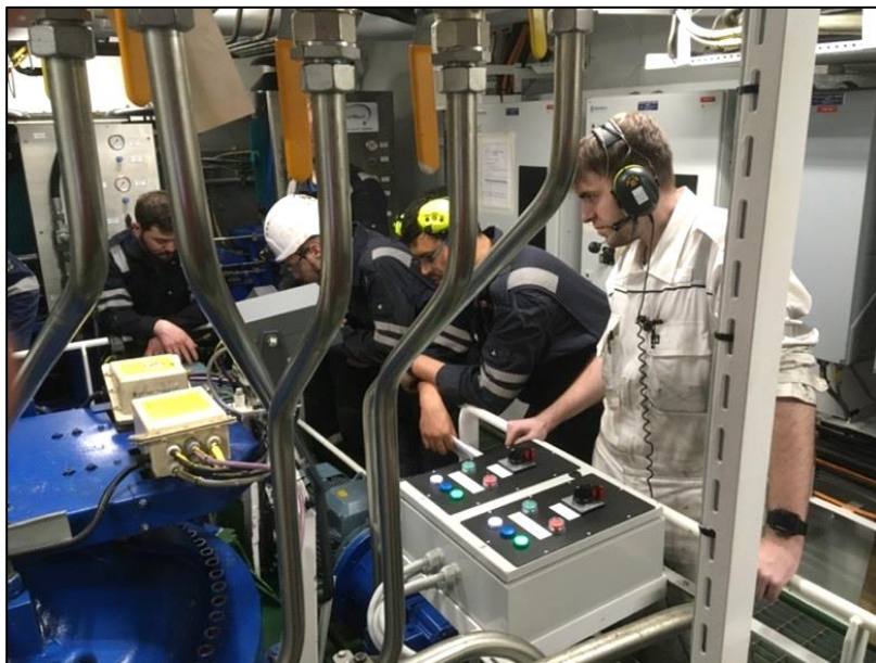
Fig. 2 Steering gear operation from emergency local control point
